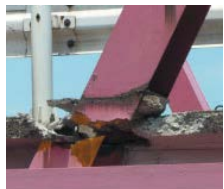
Fig. 1 Damage observed in a truss member due to corrosion. (adopted from [2])
