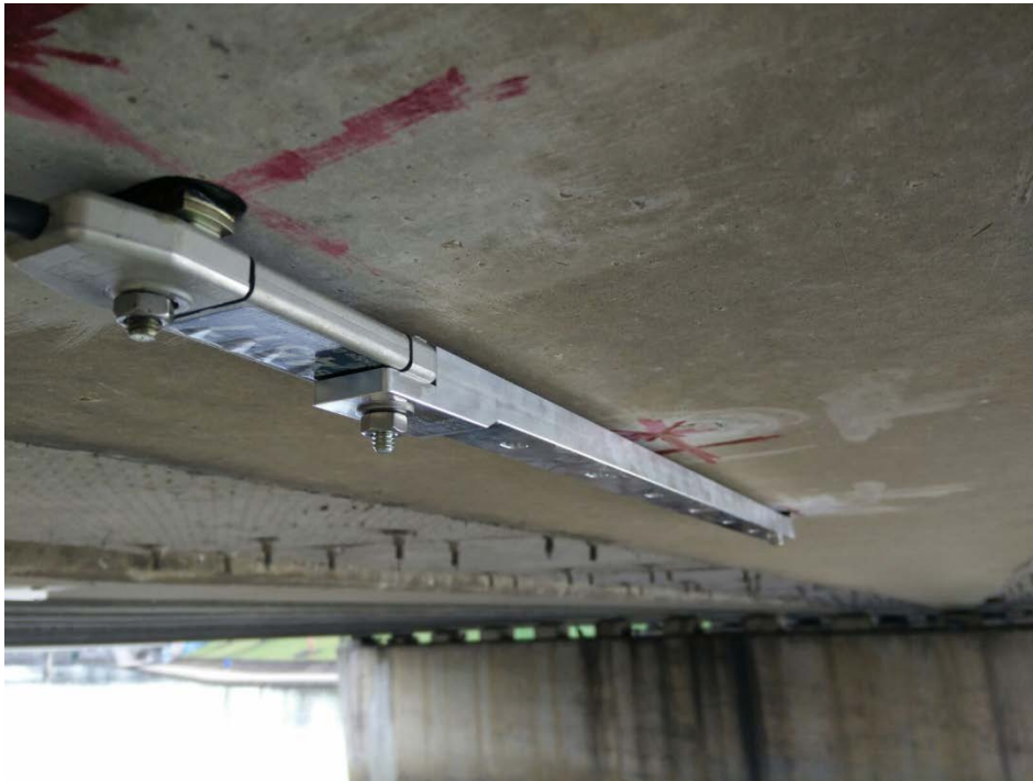
1 Fig. 3 Strain Transducer attached on a girder soffit with an aluminium extension rod
