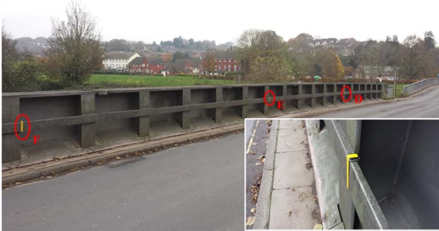
Fig. 9, IMUs deployed at sensor locations F, E & D (see Fig. 7), insert shows how IMUs were simply taped to the horizontal member adjacent to the vertical web stiffener.
