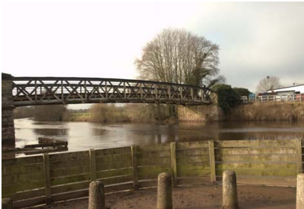
Fig 15 Side elevation of Verners Bridge. (Image taken from location of cameras monitoring deflection)
