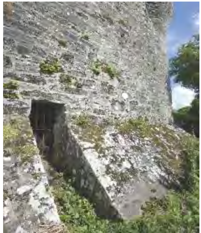
Pl. 4.21—The sally-port opening through the southern bawn wall and later wall batter, looking north-east from the lough shore (Photographic Unit, NMS).
