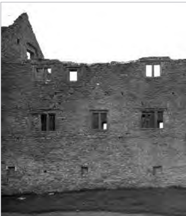
Pl. 3.12—Pre-conservation view of the exterior eastern façade of the manor house (Photographic Unit, NMS).
