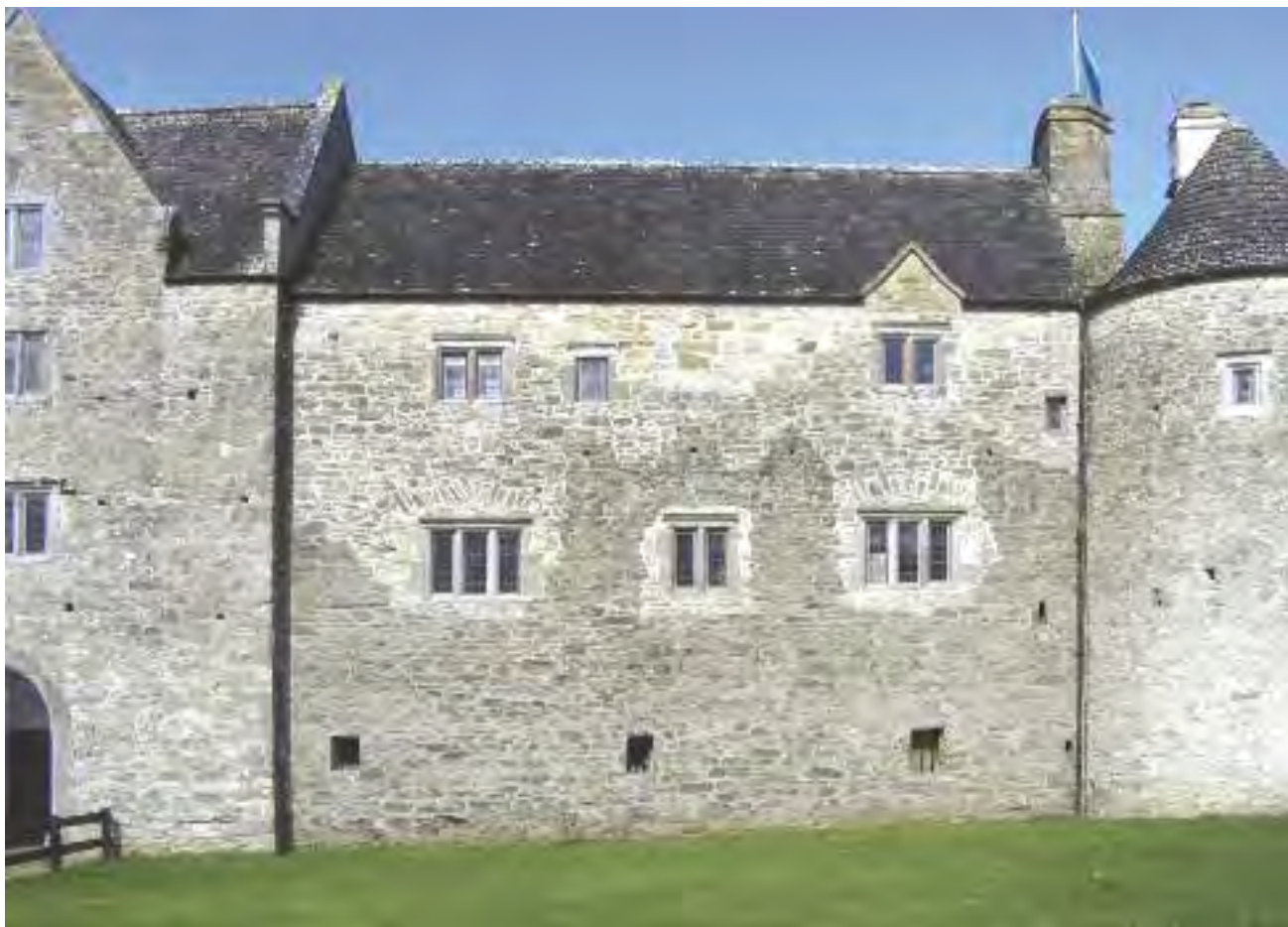
Pl. 3.14—Eastern façade of the manor house, showing evidence of the incorporation of the bawn wall into its fabric. Shading has been used to highlight the earlier bawn wall (S. Gormley).
